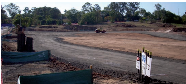
ABOVE: The site compound at Nujooloo Road is swiftly taking shape, and is expected to become fully operational in March 2010.
